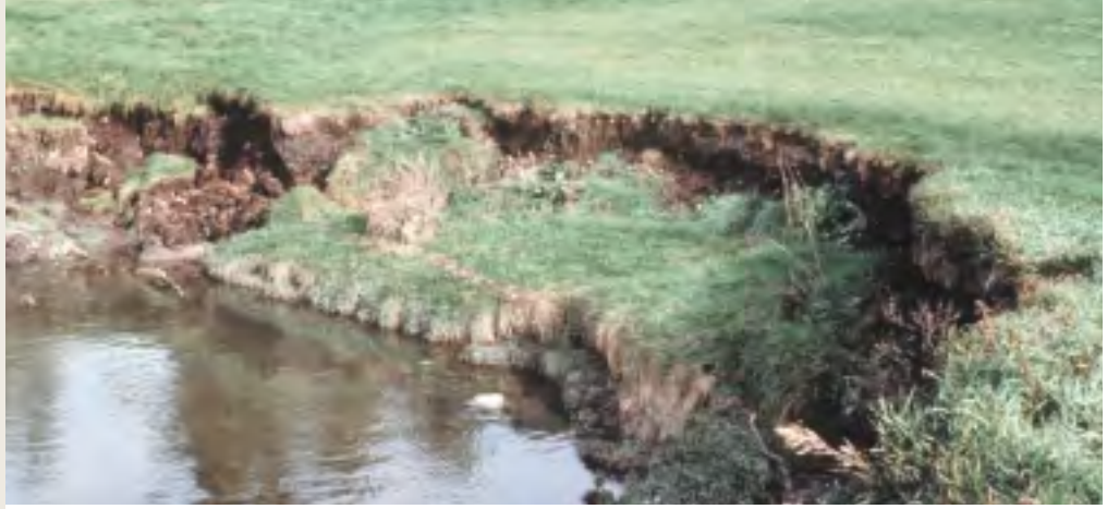
River bank erosion
