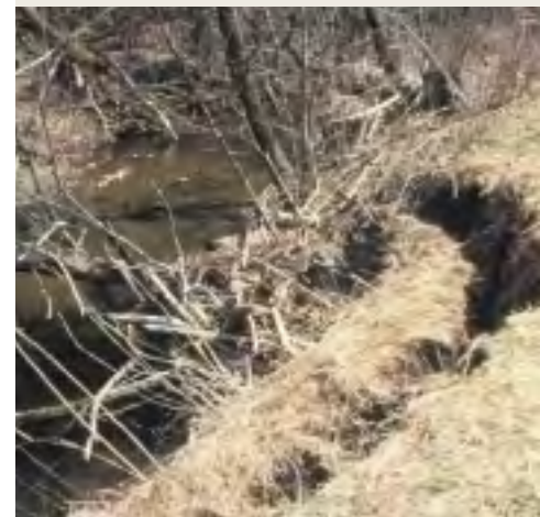
River bank erosion
